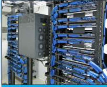
STRUCTURED CABLING SYSTEM
